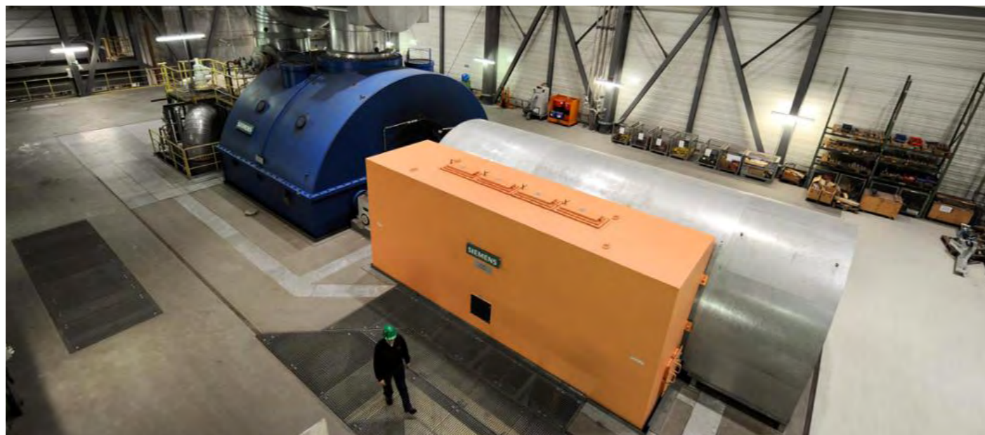
Steam Turbine and steam Gas Turbine Generator
